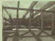
Roof repairs made to a building in Brodbeck, Pennsylvania. The roof needed replacing and the first stage of replacing the rafters took about 10 days with a group of 4 friends from NYC, 2009.
